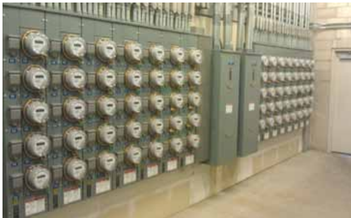
Figure 17 - Electrical room with Limited Accessibility to Individual Meters or Electrical Panels, Photo Courtesy of Todd Ritter AST
