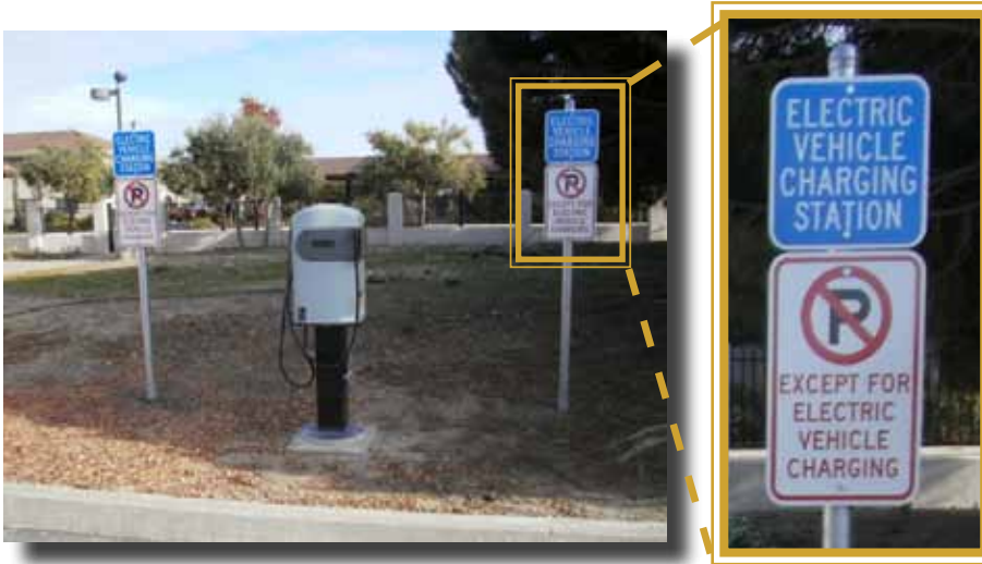
Figure 4 - Two publicly available EVCS in private off-street parking facility. IBEW offices in Castroville, CA. Photo by LightMoves Consulting
